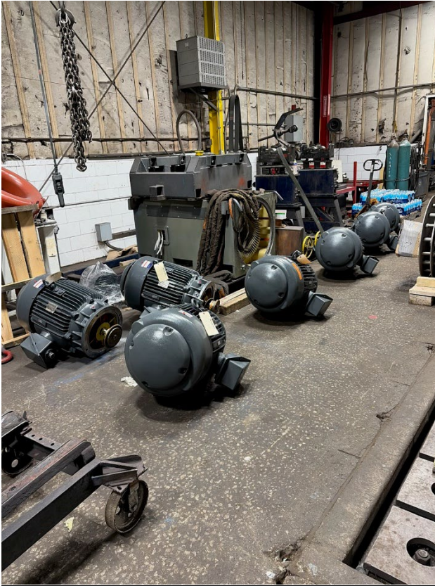
The final group of rebuilt RAS motors repaired by Bodine Electric
