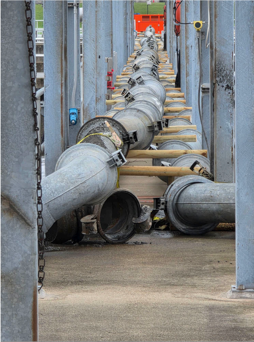
Temporary RAS Piping – (3) 12-inch pipes
