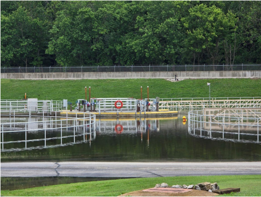
Final Clarifier Flooding
