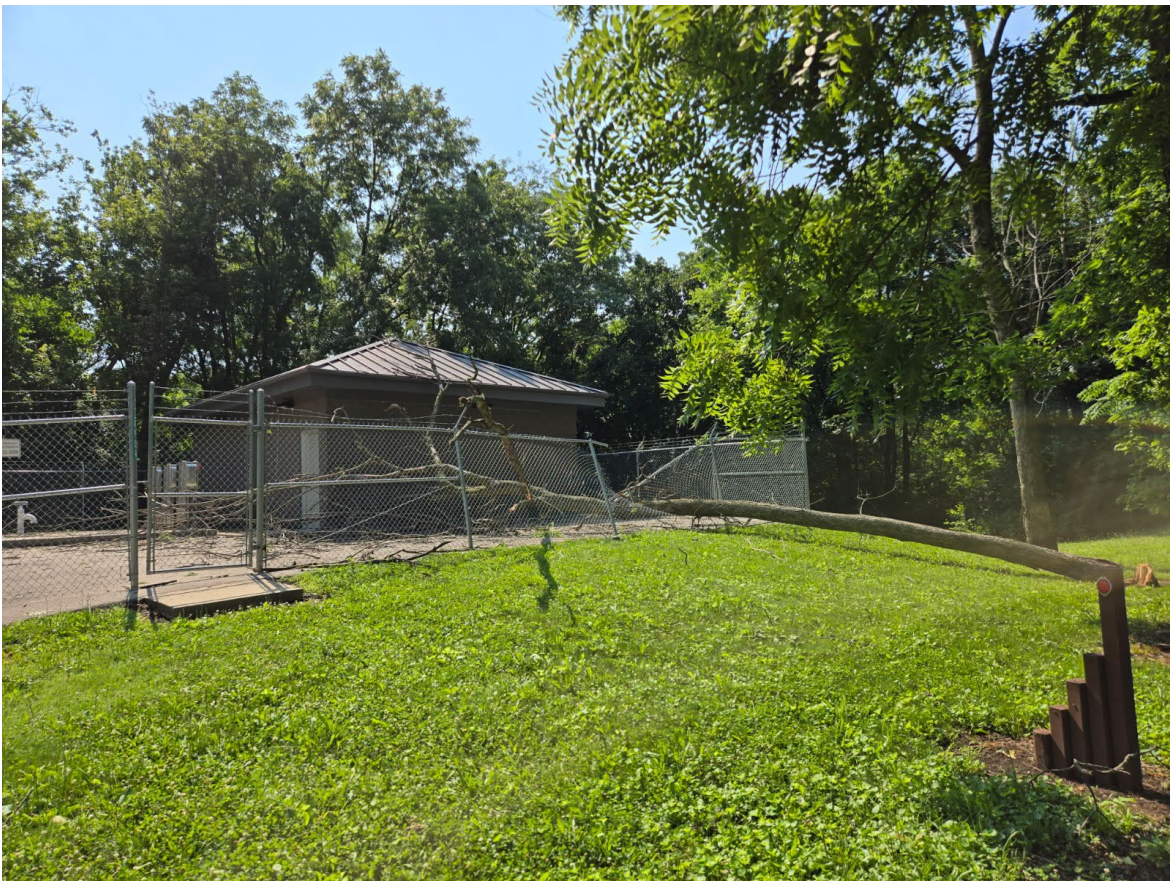
Fencing Damage – Hickory Point Pump Station
