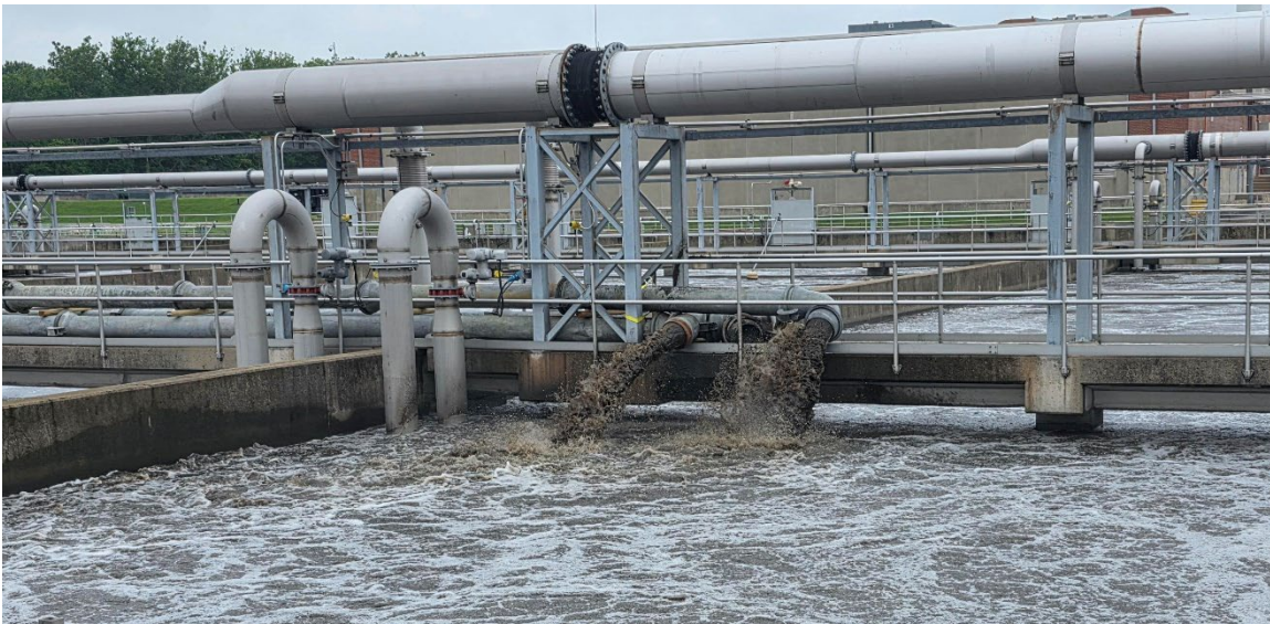
Temporary RAS System in operation – Approximately 14MGD
