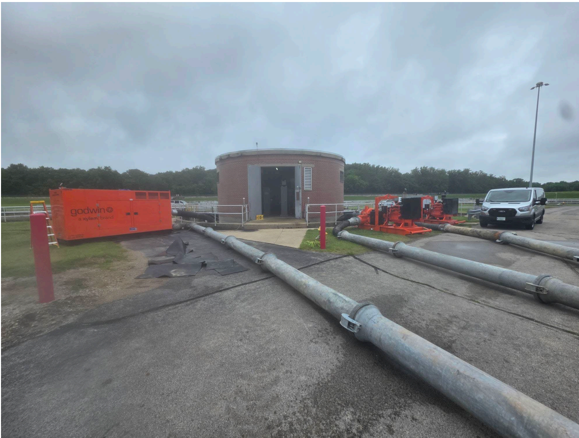
Temporary RAS Pump Setup
