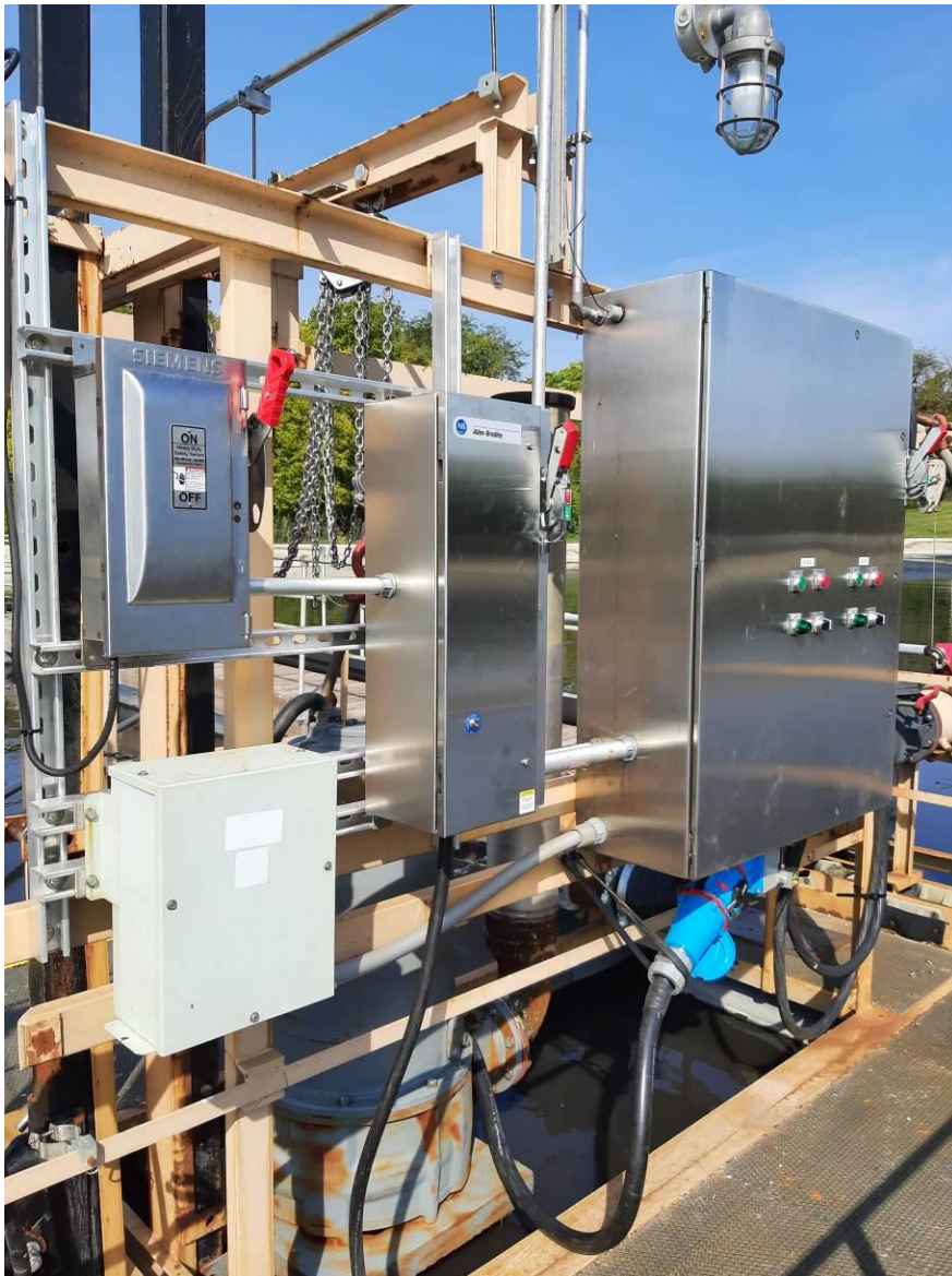
Replacement Wyckles Loadout Barge Control Panel and Disconnects
