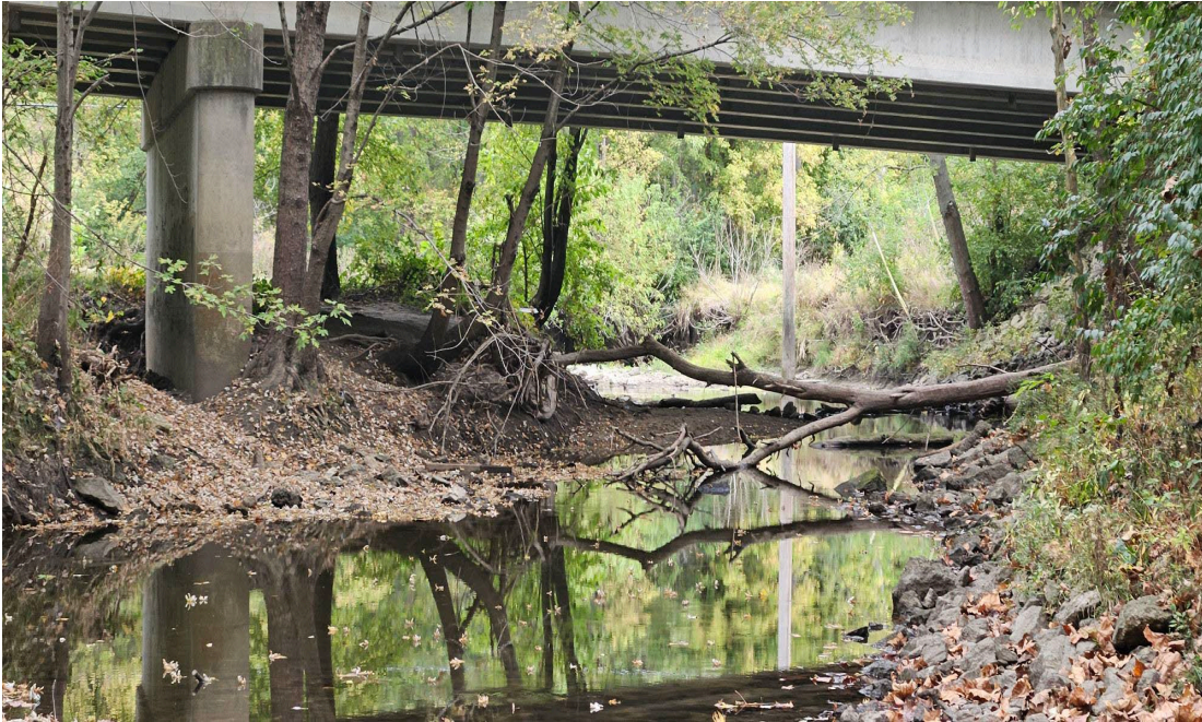
Stevens Creek Trestle – Looking North – Before – Erosion on trestle supports and fallen trees in the creek.
