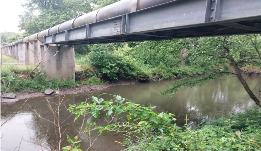
Stevens Creek Trestle – Looking East – Before – Trestle supports at risk. No erosion control on the creek banks.
