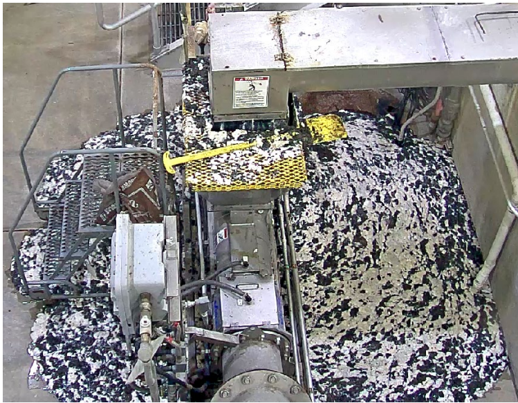
Photo 3: Overflow reaching edge of stairs
